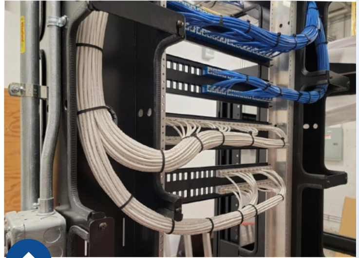
Neatly dressed voice and data cabling connected into the back of patch panels.
